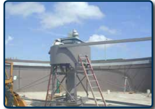
IN PROGRESS: This project resurfaced outer and inner concrete walls and replaced the internal equipment, bridge, peripheral walkways, air header, skimmer arm, feedwell, drive, weirs, and control panel.
