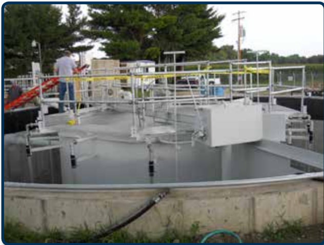
IN PROGRESS: Splitter Box, air header, drop pipes, diffuser assemblies, walkways and controls were replaced.
