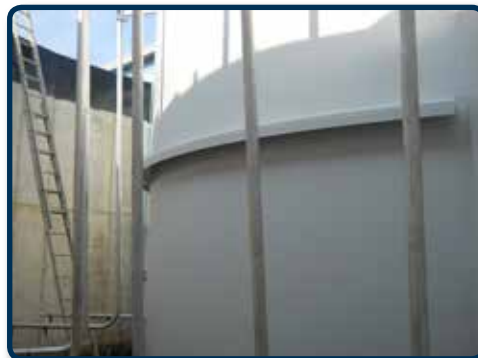
AFTER: New reinforcing ring added to clarifier tank and the tank was recoated. Also as part of the retrofit project, the air header, blowers, drop pipes and diffuser assemblies were replaced.
