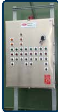
AFTER: Controls were replaced and now tie into district's new SCADA system.
