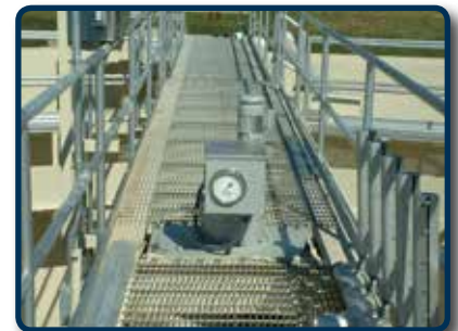
New Clarifier Drives
