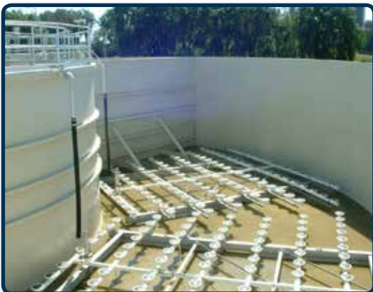
AFTER: Reinforcing rings were added to the clarifier for dewaterability. A new partition, reinforced knee braces and new inlet box were added.
