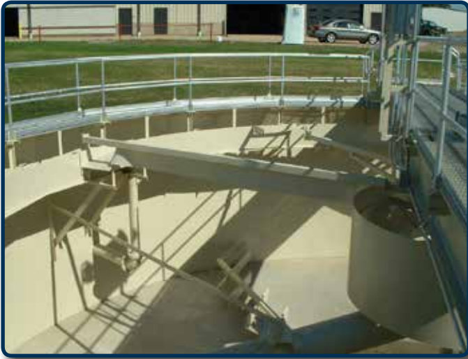
AFTER: Walls were resurfaced and painted and the scraper arm, skimmer, feelwell, and drive were replaced.
