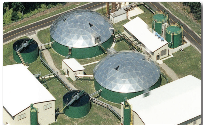
(Pictures above) At this field-erection site, Smith & Loveless coordinated its work with other contractors and crews on-site. They all meet their critical deadline—complete field-erection, installation and start-up in less than three months.
