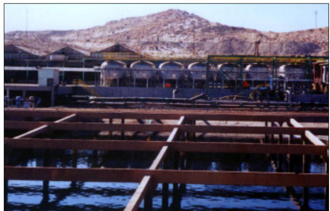
The Andes Mountains surround the seven S&L DI-SEP® SX Electrolyte Filters at the Cerro Verde Copper Mine (top) located near Arequipa, Peru. These filters remove virtually all impurities allowing for the production of 99.99% pure copper plate.
